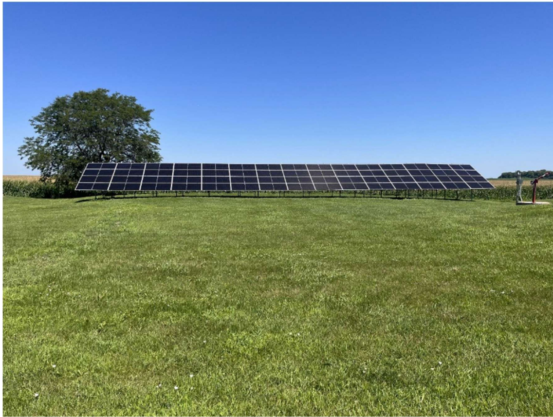
Solar system at Comfrey Wastewater Treatment Plant (Photo by Comfrey Mayor, Gary Richter)
